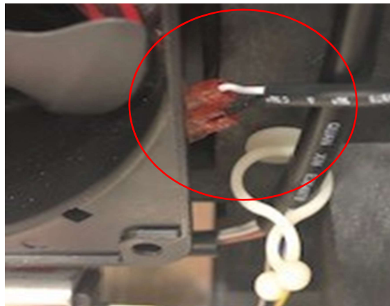
Figure 20. Terminals connected to fan.
