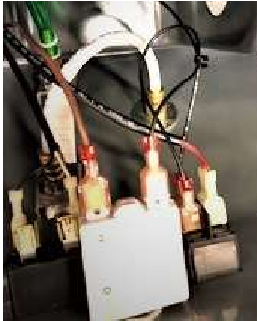
Figure 25. Showing how the front panel is wired up.
