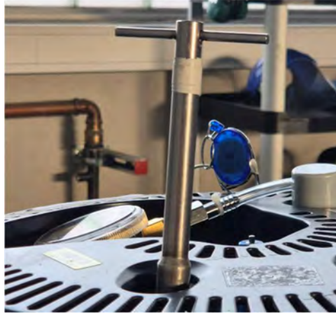
Figure 9 – Vent valve wrench fitted
